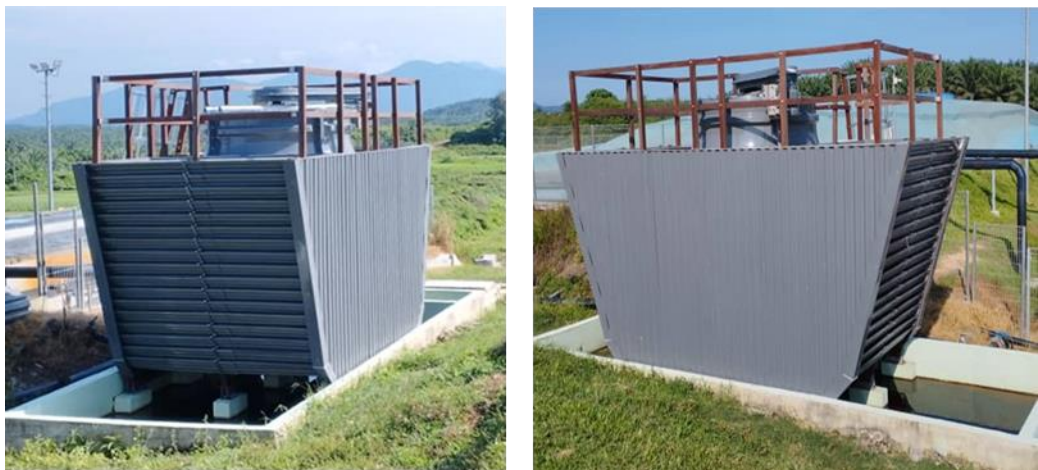
Figure 3.9: CT installed at BGP A
