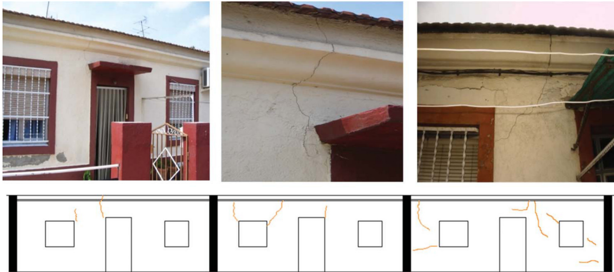
Fig. 2.27. Photographs of damage in buildings due to tunnelling (Camós et al., 2014)
