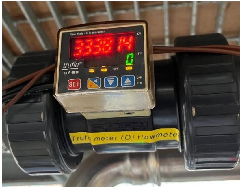
Figure 3.10: A Paddle wheel flowmeter for silicone oil flow rate measurement
