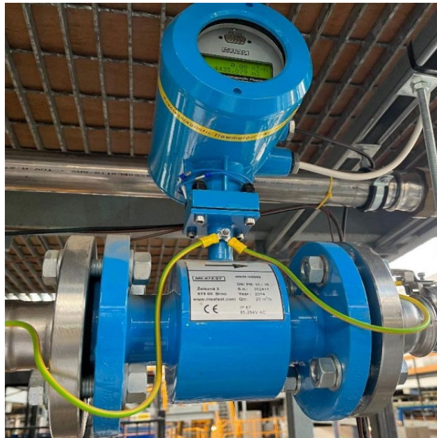
Figure 3.9: Electromagnetic flowmeter for water flow rate measurement
