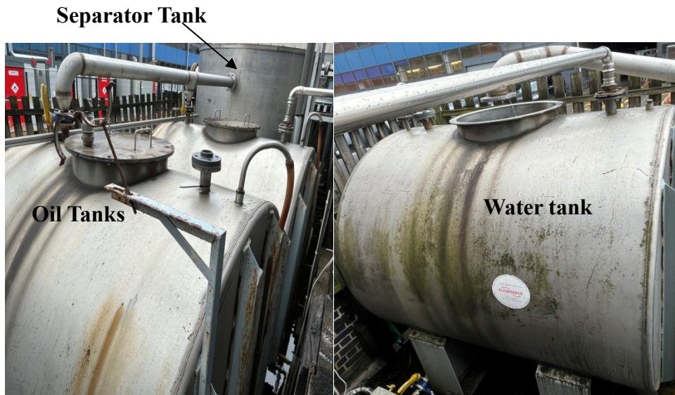
Figure 3.5: Fluid storage tanks showing the separator tank, oil tanks and the water tank
