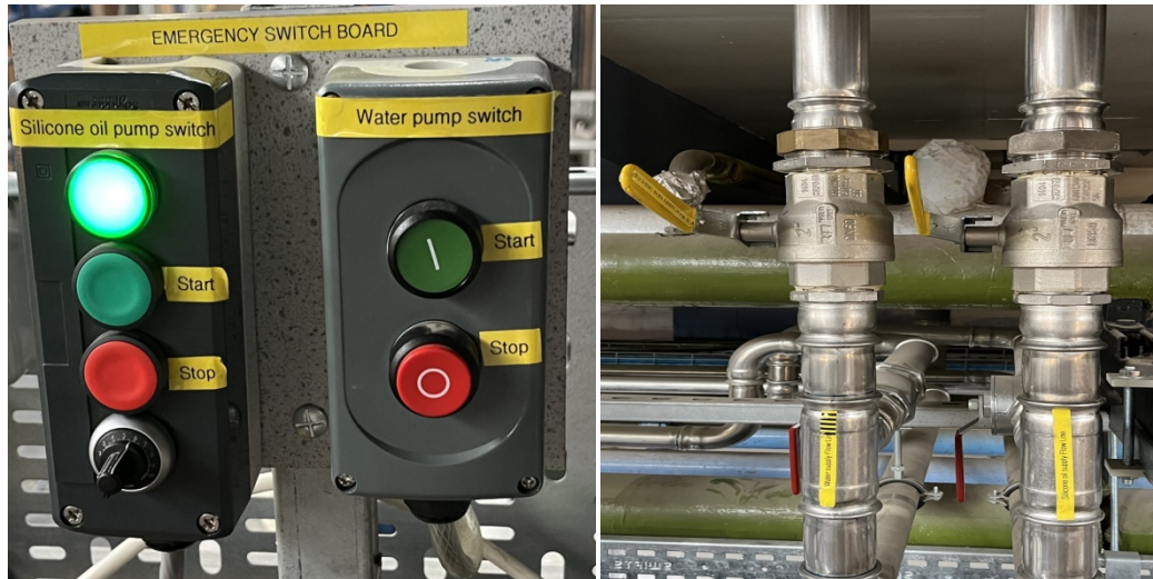
Figure 3.6: Components of the control system which includes the pump switches and the gate valves.
