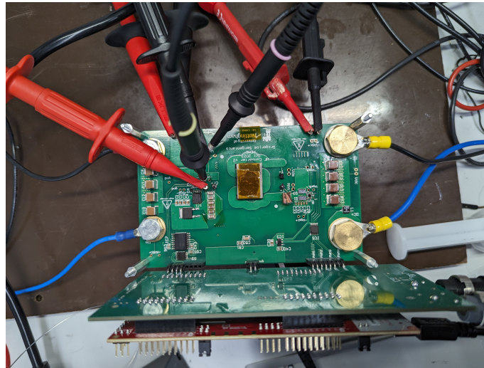
Figure 6.11: The implemented connection of the controller card.
