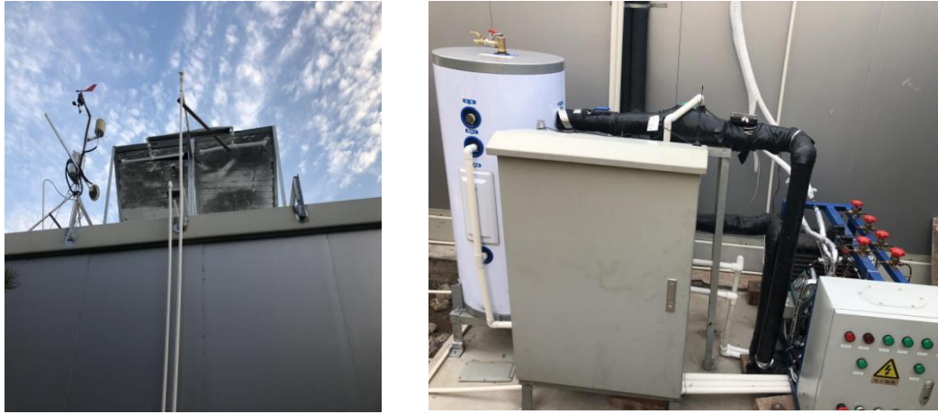
Figure 5 - 2 The picture of the part of the PV/T-ASHP system
