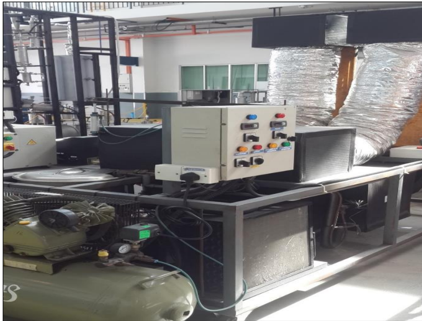
Figure 3.4 Heat pump drying system
