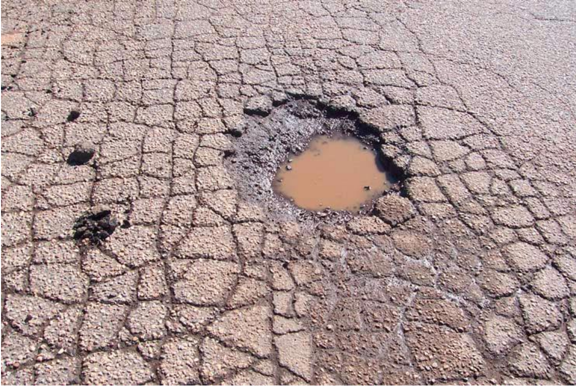
Figure 2-21 Pothole Surrounded by Alligator Cracking (FHWA, 2009)
