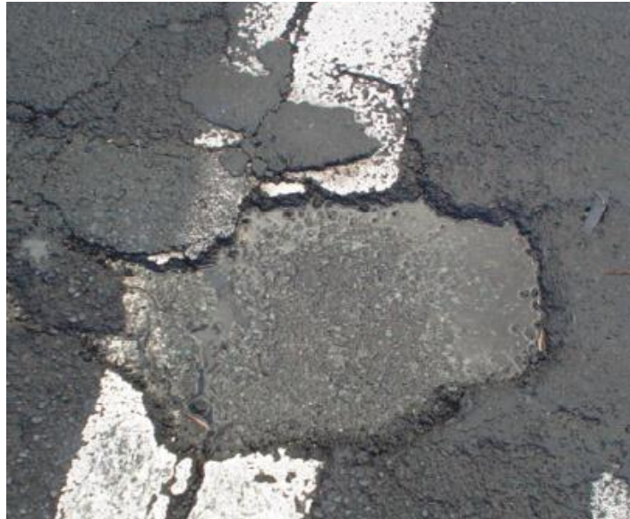
Figure 2-16 Shallow potholes caused by de-bonding (Muench et al., 2008)
