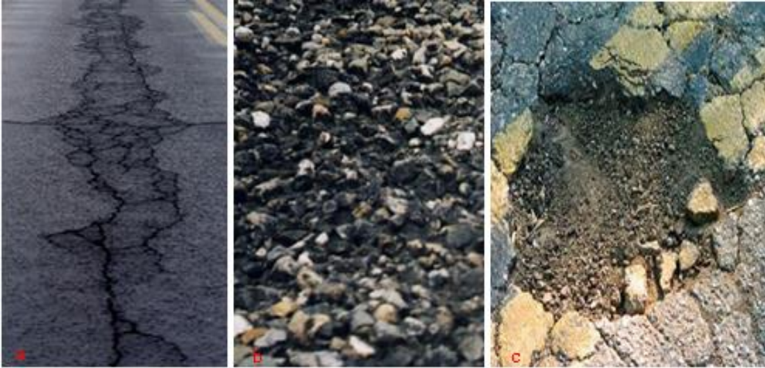
Figure 2-6 Moisture induced damage in asphaltic pavements. (a) Stripping, (b) Raveling, (c) Pothole formation (Kringos et al., 2007).
