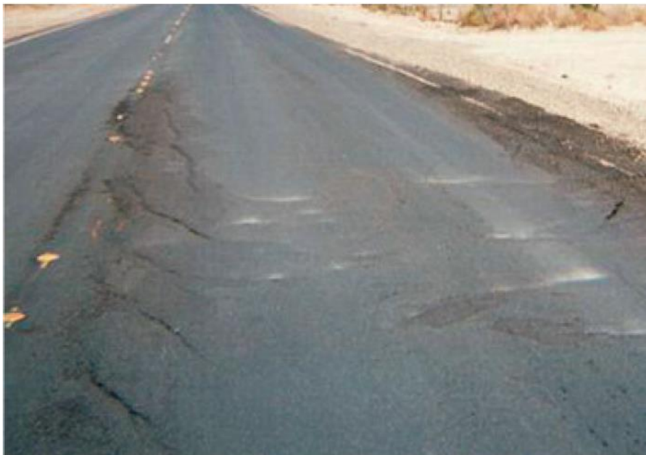
Figure 2-14 Premature slippage failure on an overlay project in Nevada, USA (Charmot et al., 2005)
