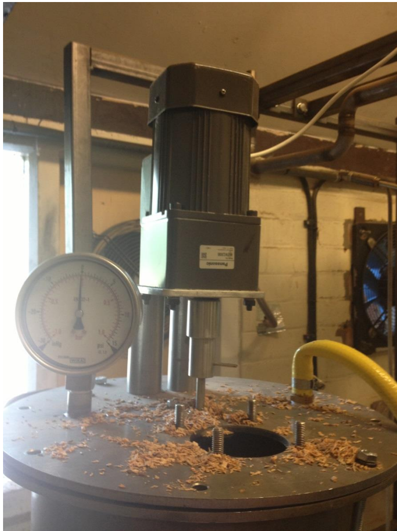
Figure 3-2: Stirrer and pressure gauge installed at woodchips hopper
