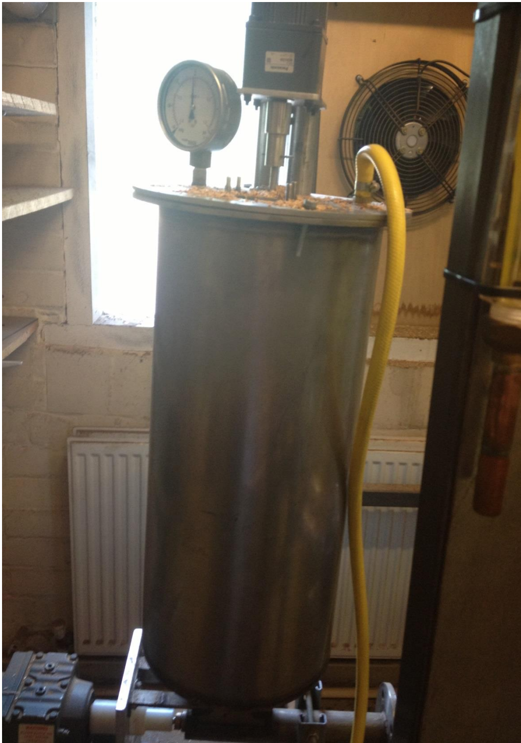
Figure 3-4: Cylindrical shaped woodchips feeder hopper.
