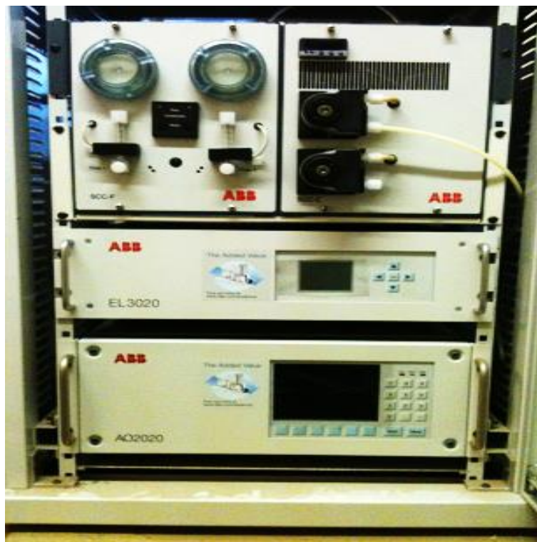
Figure 3-14: ABB online gas analysers equipped with sampling unit.
