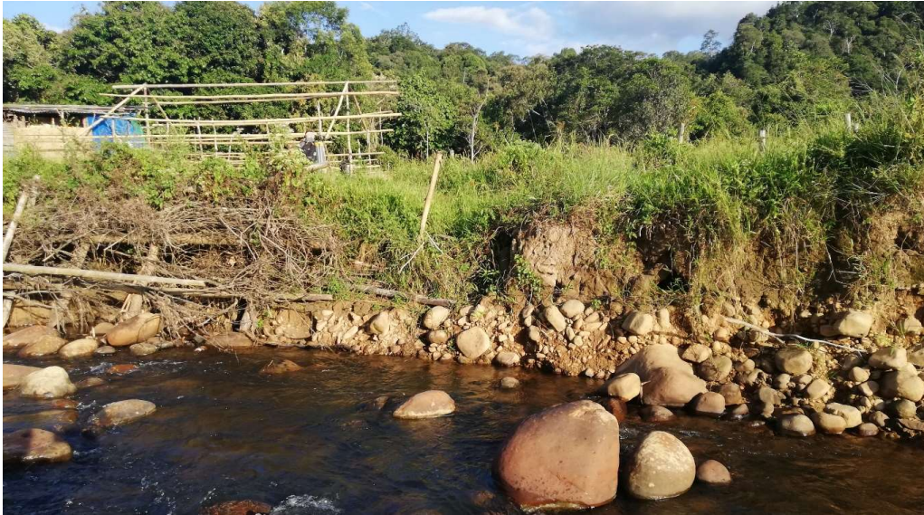
Plate 4.6: Eroded bank after brush wall was washed away in December 2019 at Site A.
