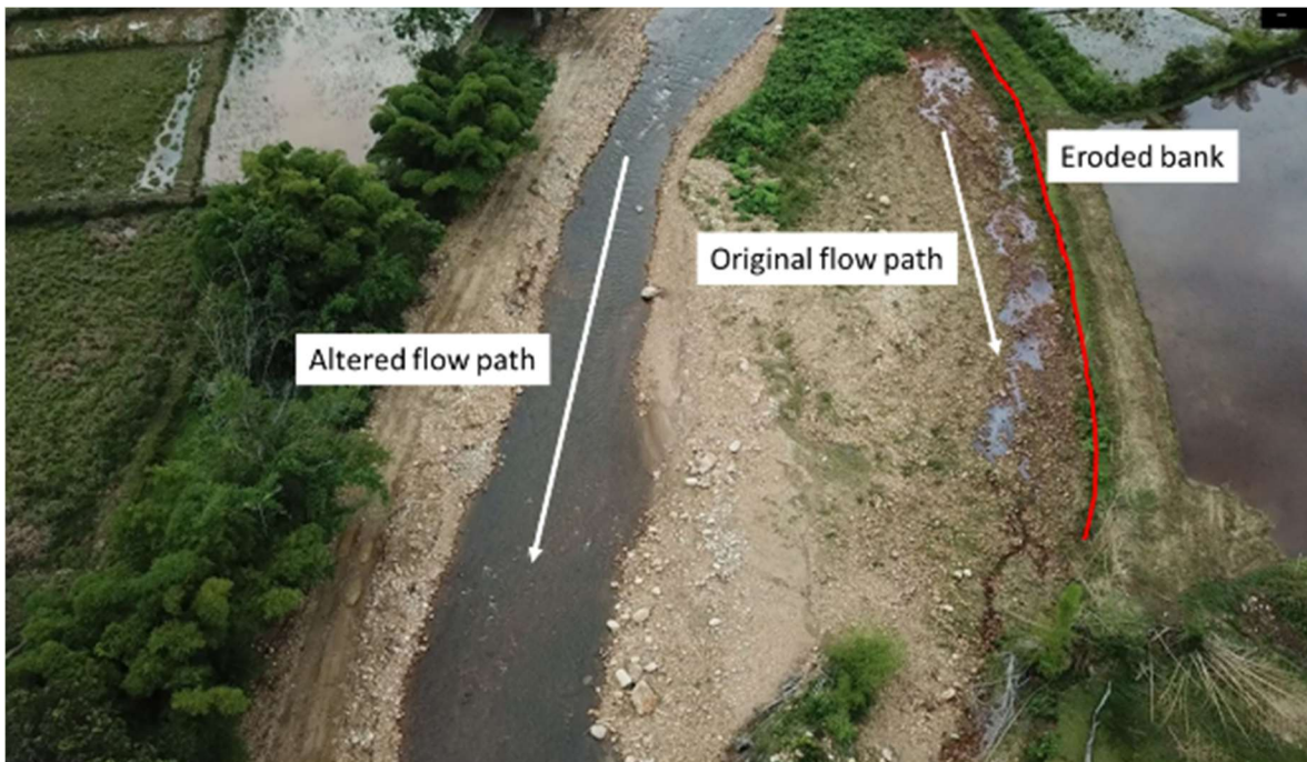
Plate 1.1: Channelised reach at Long Semadoh with large gravel shifted from the true right bank to the true left eroded bank.
