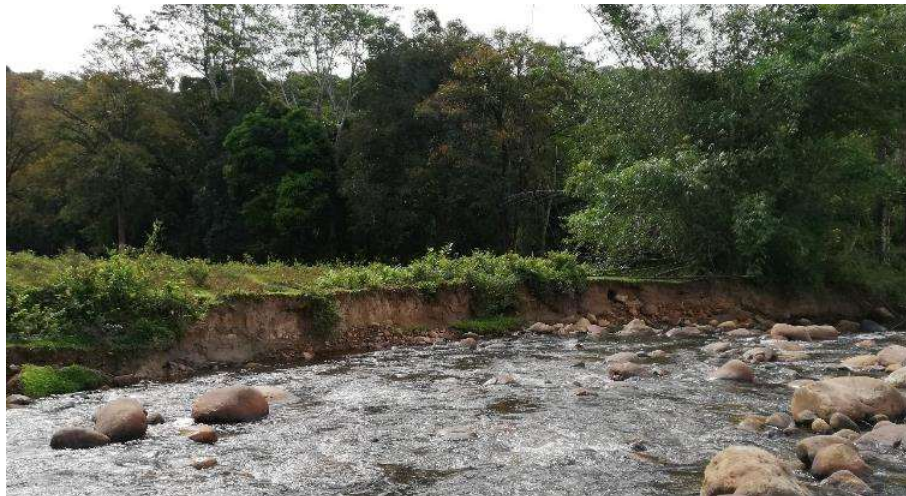
Plate 4.11: Eroded bank (soil fall) at the lower section of Site B.
