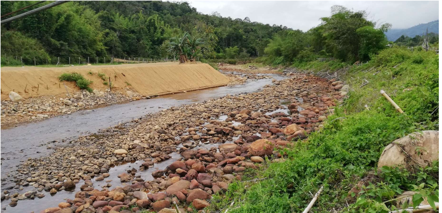
Green bank protection measures installed near Long Telingan Photo: Yih Yoong Lip, February 2021
