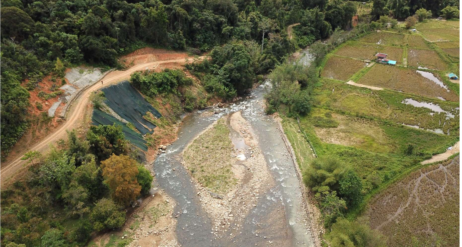
Landslide area and gabions at the Upper Trusan River Photo: Yih Yoong Lip, February 2023
