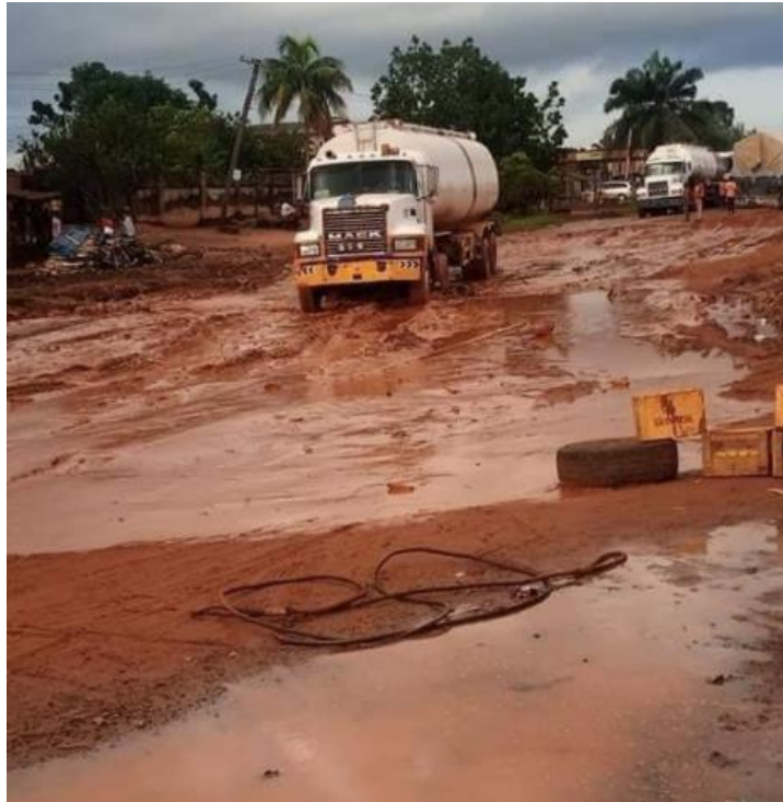
Figure 6.21: Bad roads in Nigeria
