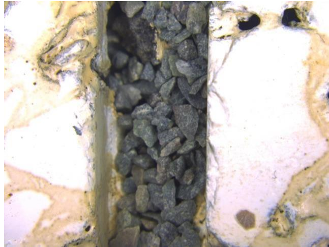
Figure 72. Image of detritus within a crack
