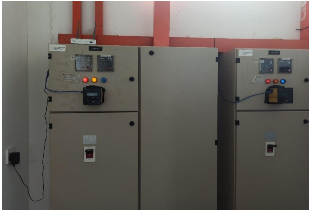
Figure 3.5: ION 7330 meters and the wireless router in SSB room
