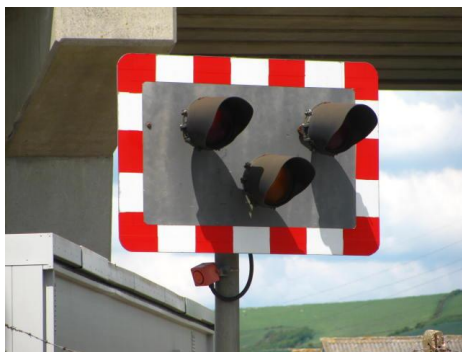
Figure 4-8 Wig-Wag Road Traffic Lights.
