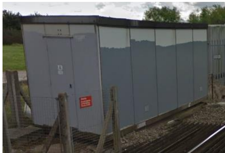
Figure 4-12 Road side cabin containing the control system - mismatched paint indicating a repair has taken place.
