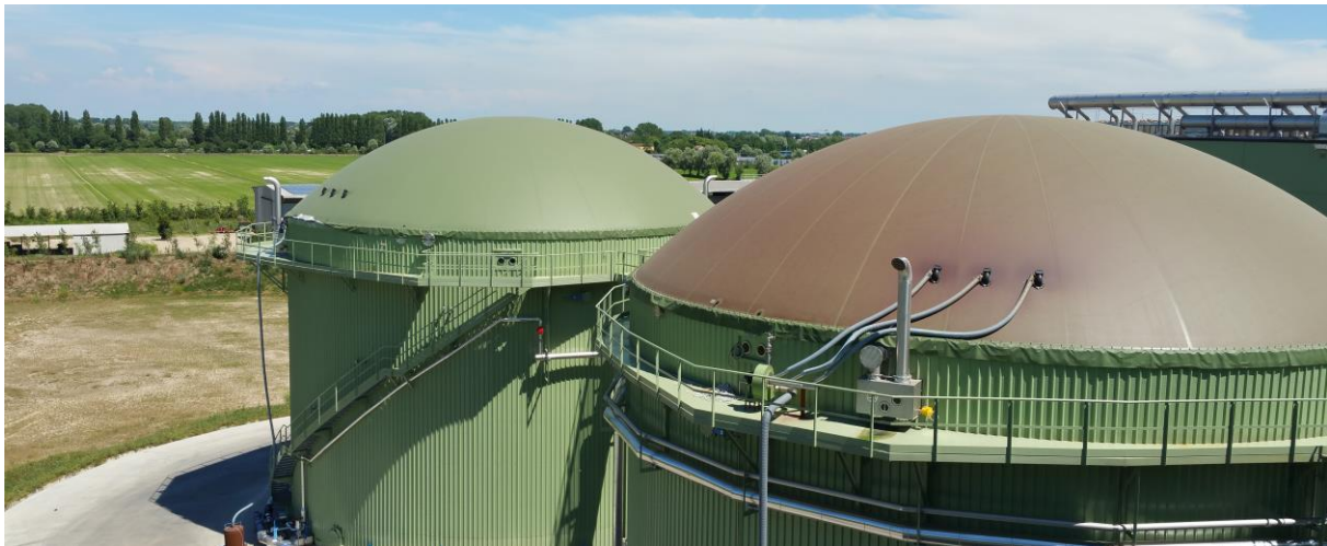
Figure 2: Typical double layer pneumatic roof for digesters. The change in the colour of the membrane roof it is clearly visible and it is related to the degradation of the membrane due to the aggressive chemical environment. (source: Maco Technology srl).
