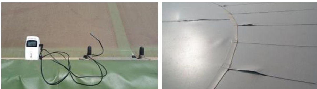
Figure 7: Damages to the welded seams due to the high temperature that during a sunny day in the warm season reaches 66.5°C (source: Maco Technology srl).
