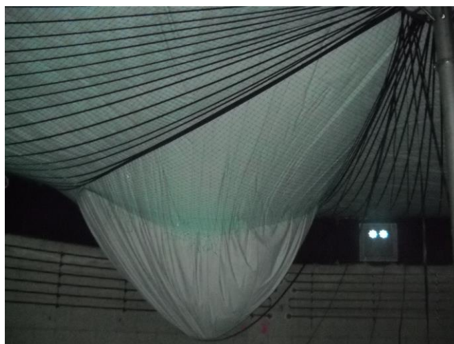
Figure 9: Failure due to snow load (source: Maco Technology srl).
