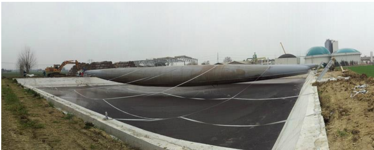
Figure 3: Rectangular lagoon covered with a pneumatic beam [5] derived from the Tensairity® concept with a total span of 45m (source: Maco Technology srl).
