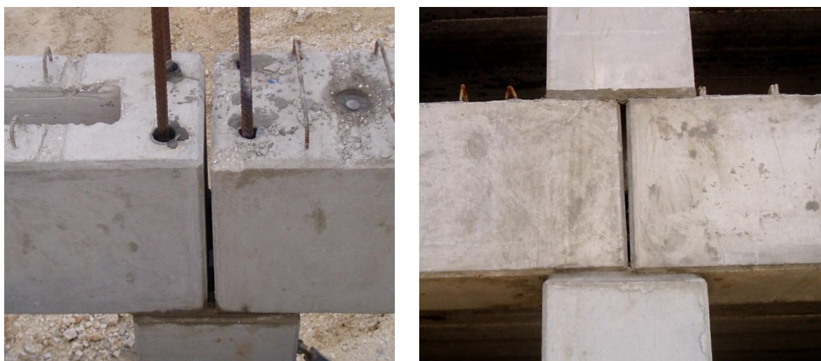
Figure 1.1 Discontinuous beam-column connection used in a braced frame car park project – Preconco Ltd., Barbados, 2010
